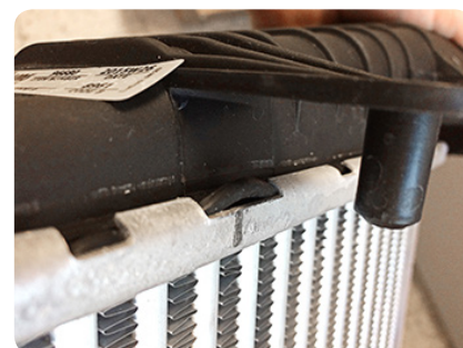
A too high system pressure can cause deformation of the plastic tank.
